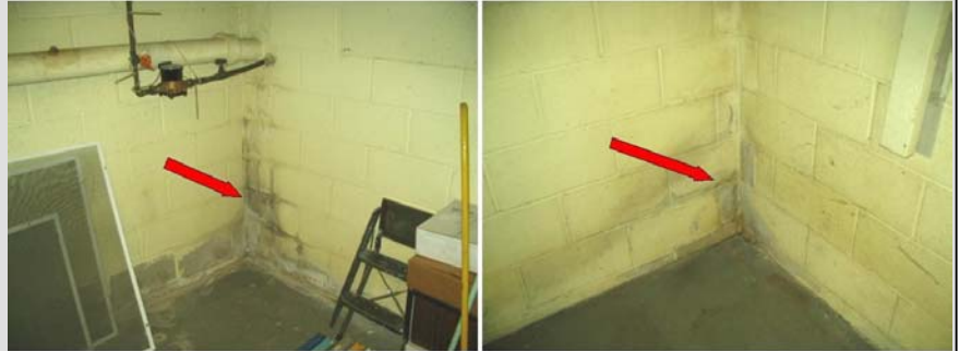
Staining in corners indicates periodic moisture.
