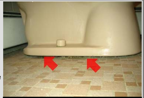
Loose toilet due to raised flange
