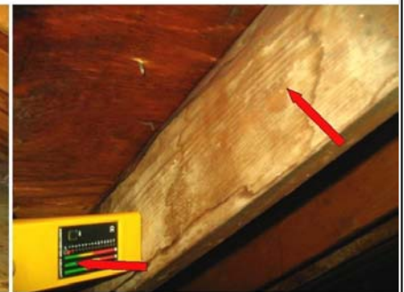
Stains on framing was dry.
