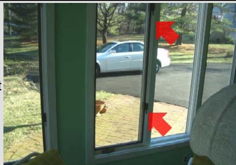
Window is difficult to latch
