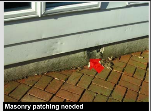
Masonry patching needed
