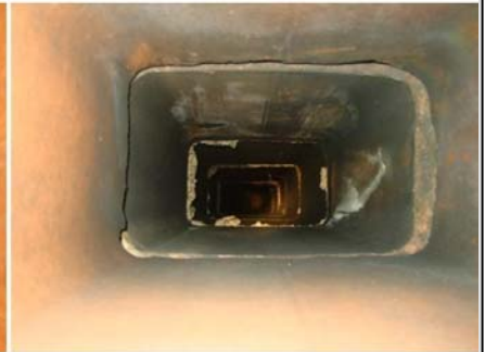
Inside of fireplace liner.
