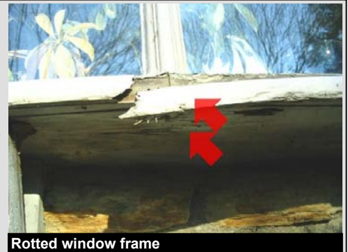
Rotted window frame
