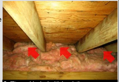
Soffits are blocked with insulation
