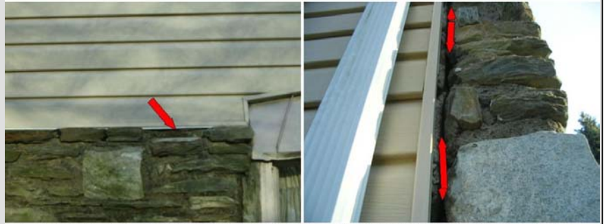
Repair missing stone at front of house. Sealant needed where vinyl siding meets stone.
