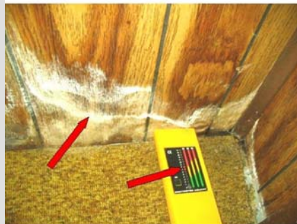
Staining and elevated levels of moisture present on paneling.
